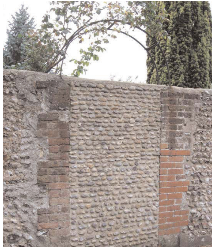
Fig. 9 - Blocked entrance to walled garden
